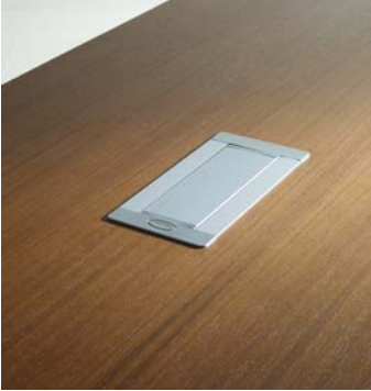
Electrical Detail Closed
