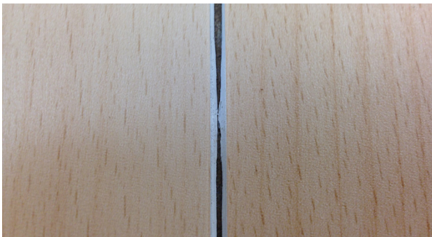
This seam has been grooved too deep. This will result in seam failure over time.
