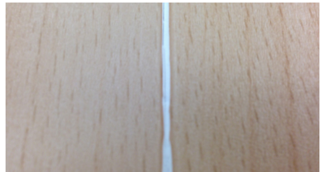
This seam has not been grooved deep enough. This will result in seam failure.
