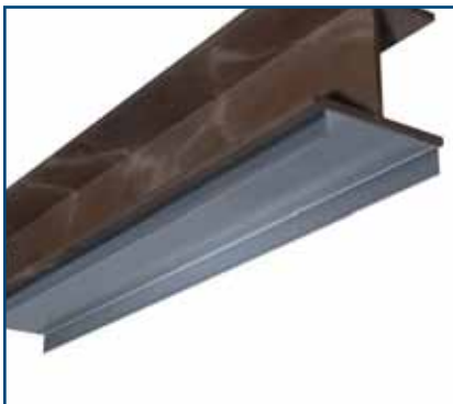
Attach 20ga standard leg track to structure. Track will allow for alignment and closure.
