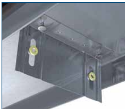
Fasten SL to top track at designed stud spacing with engineered fastener.
