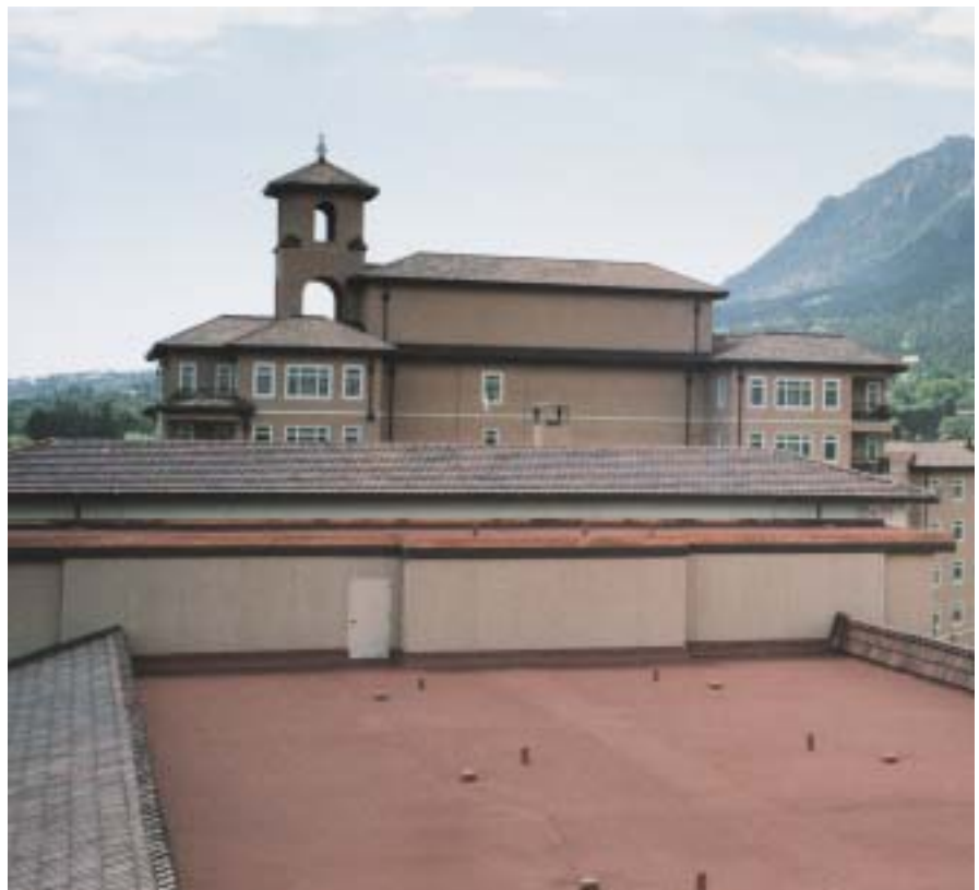
After the previous roof membrane was removed from the five-star Broadmoor Hotel in Colorado Springs, 1/2-inch DuraBoard insulation was applied. Two plies of APP modified bitumen were then heat welded to the perlite board without the need for an additional base sheet. (Photo courtesy of Johns Manville, Denver.)
